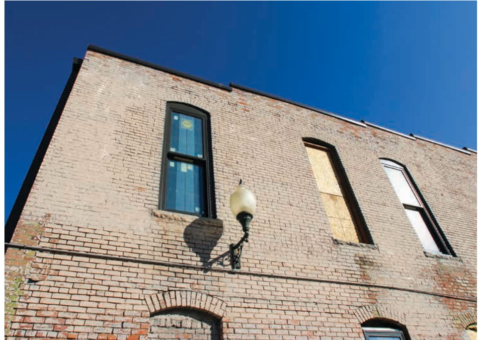
Lacy Construction is part of the team chosen to remodel a 115-year-old, two-story brick structure in downtown Grand Island.
